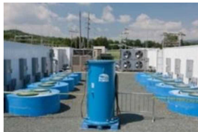
20MW/5MWh Flywheel/Beacon Power (ニューヨーク州; Flywheel Frequency Regulation Plant)
