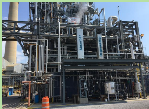
Slipstream Solvent Test Unit
