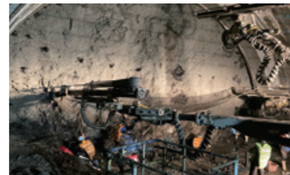
Conventional explosive loading and wiring. The operator loads the explosive and connects the wire directly under the excavation face where concrete is sprayed while implementing safety measures such as rockfall protection nets, etc. It is required to make the operation remote so as not to be involved in a disaster such as a landslide during the operation.
