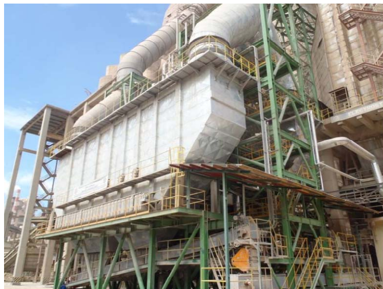
Additional SP boiler
