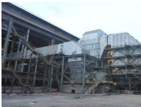
Waste heat recovery equipment
