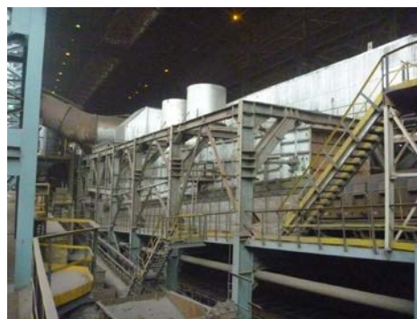
Heat recovery hood
