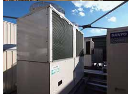
Test site: MaxValu Express Rokugodote Ekimae Refrigerator showcase Non-fluorinated refrigeration system installed on store roof
