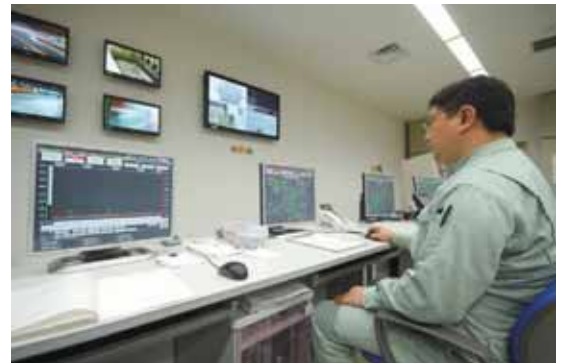
Control room at the Kunisaki Clean Center
