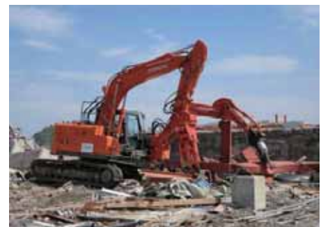
Metal scraps from construction structures and foundations complicatedly intertwined with each other were finely cut and separated to be transported. (Minami-Sanrikucho)
