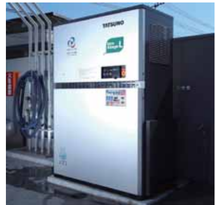
The Eco Stage L liquefies and collects gasoline vapor that is generated when unloading the gasoline from a tanker truck into an underground tank.
