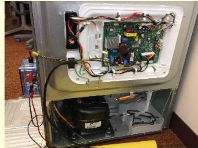
Refrigerator, 380 V DC, 1% W saved (since original doesn't have PFC)
