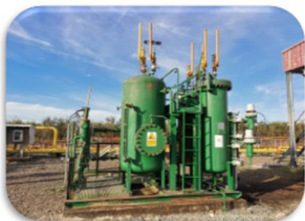
4. Fuel Gas Unit
