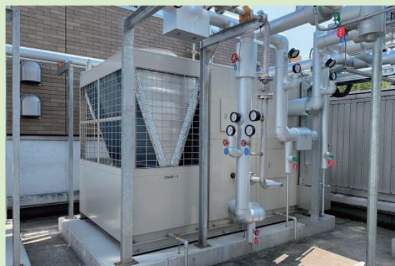
▲ Heat pump demonstration system
