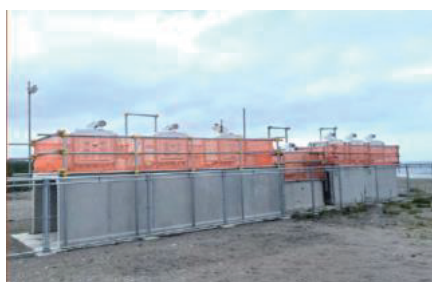
▲Platform for the installation of the Doppler lidar
