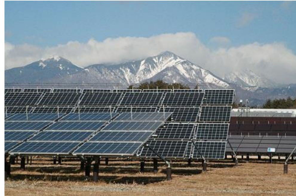
Mega-solar system in Hokuto City, Yamanashi Prefecture (demonstration experiment by NEDO)
