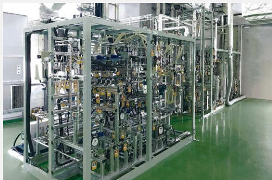
Figure 1 Pilot plant in the Chiyoda Koyasu Research Park
