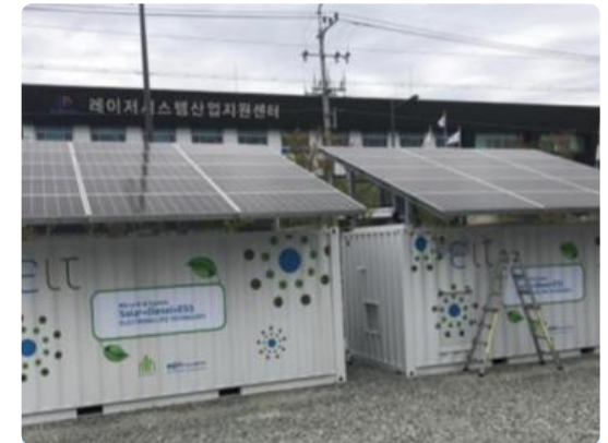
Higatangan micro-grid project
