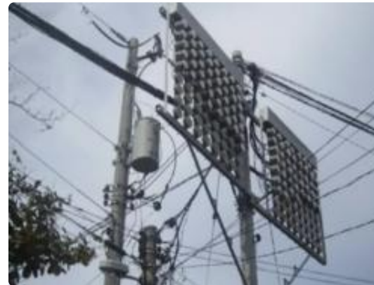
Elevated meter clusters
